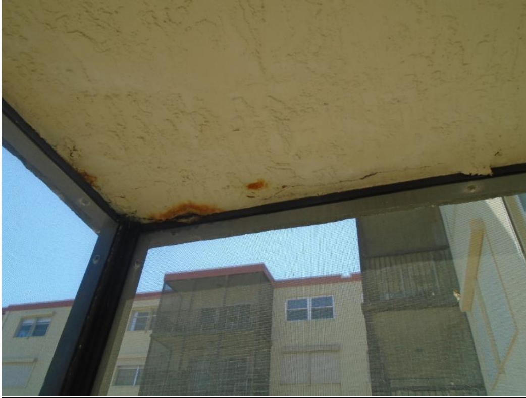
Example view slab edge Concrete spalling due to reinforcing steel corrosion
