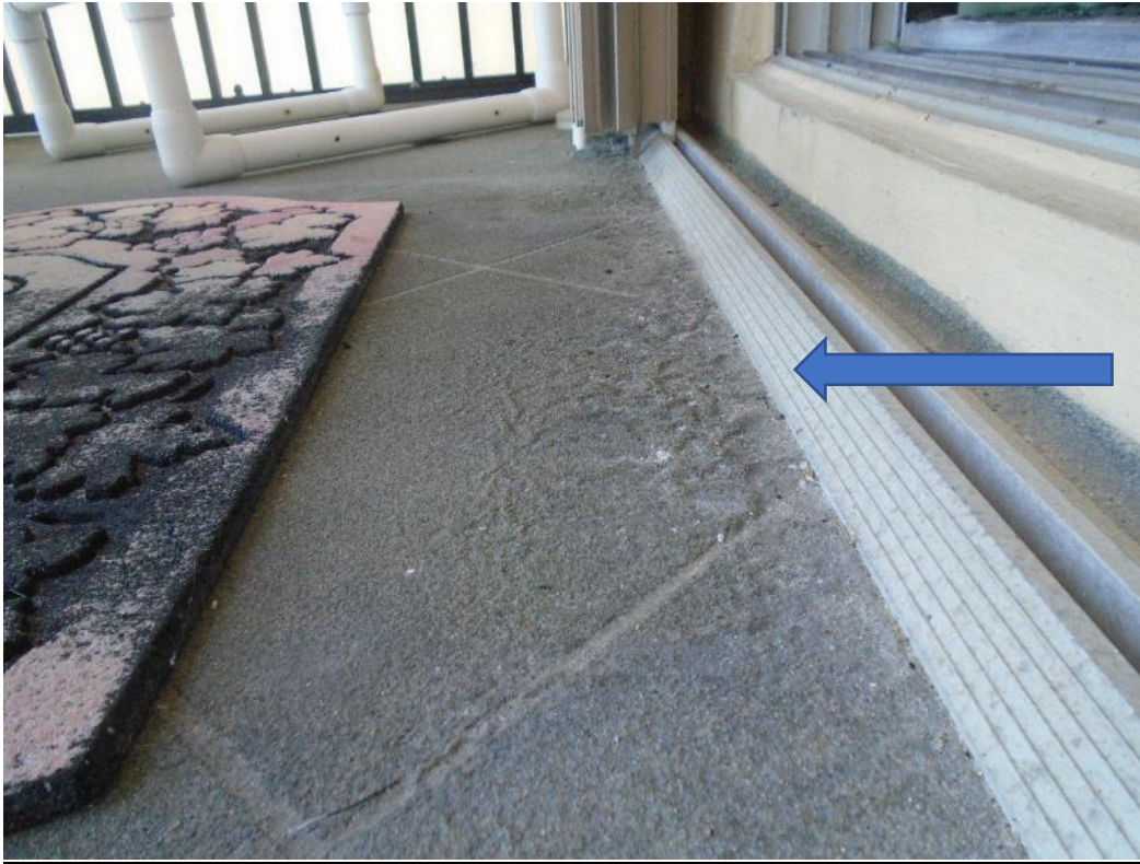
Example view of lack of drainage at shutter track resulting in floor coating failure
