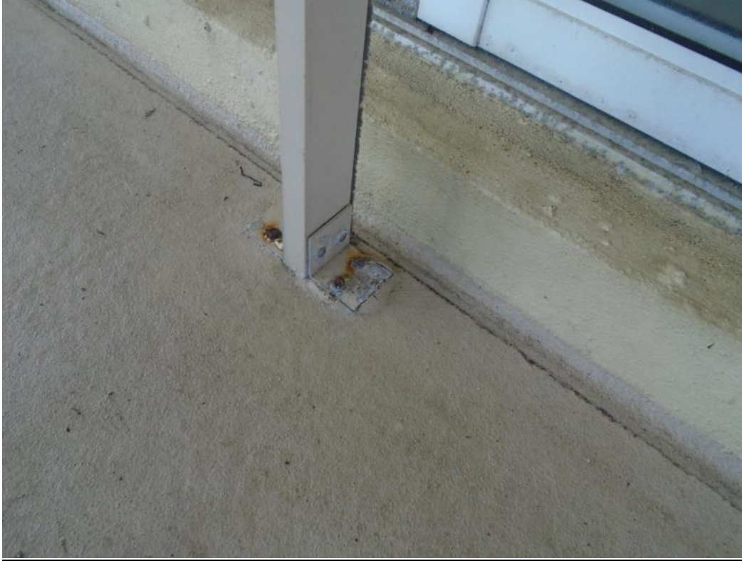
Example view of miscellaneous corroded fasteners
