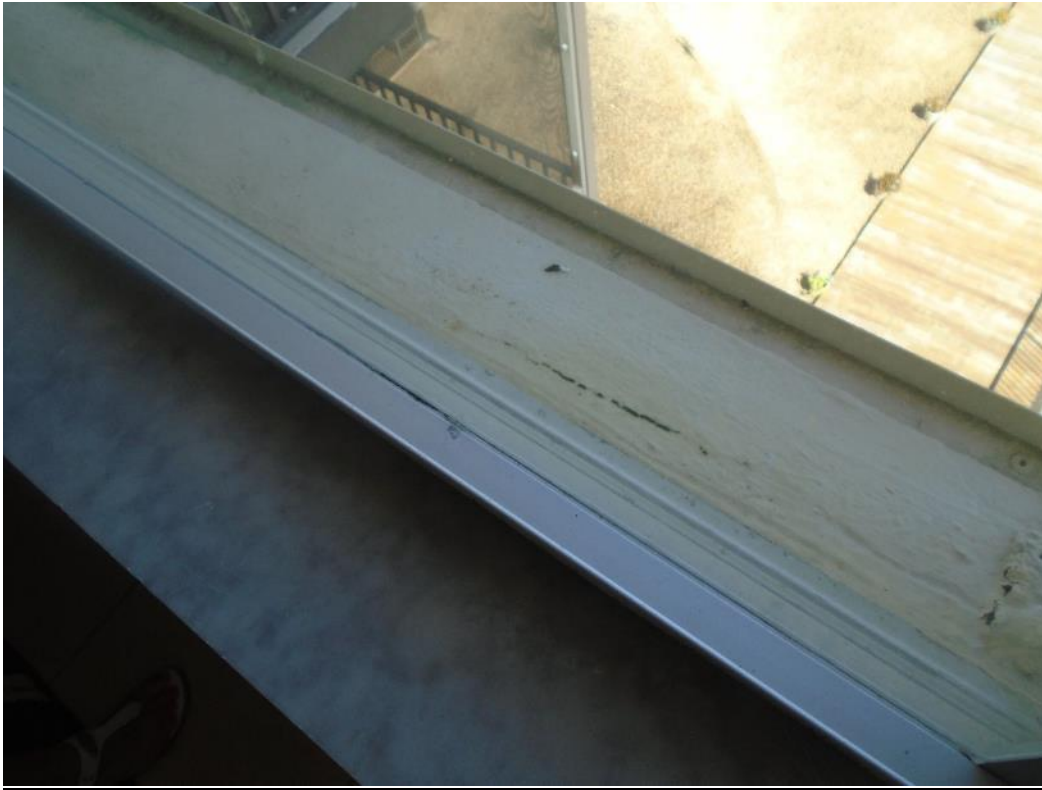
Example view Window Sill Concrete spalling due to reinforcing steel corrosion
