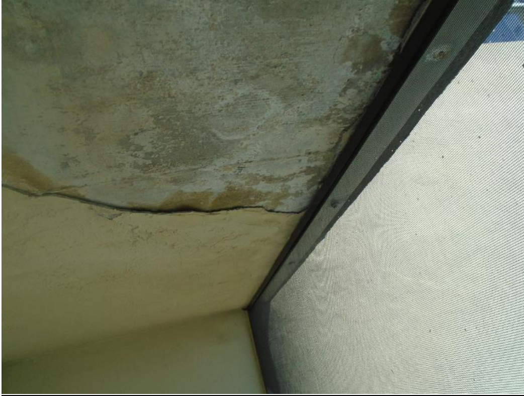
Example view of stucco loss on balcony ceiling due to poor drainage at screen frame above
