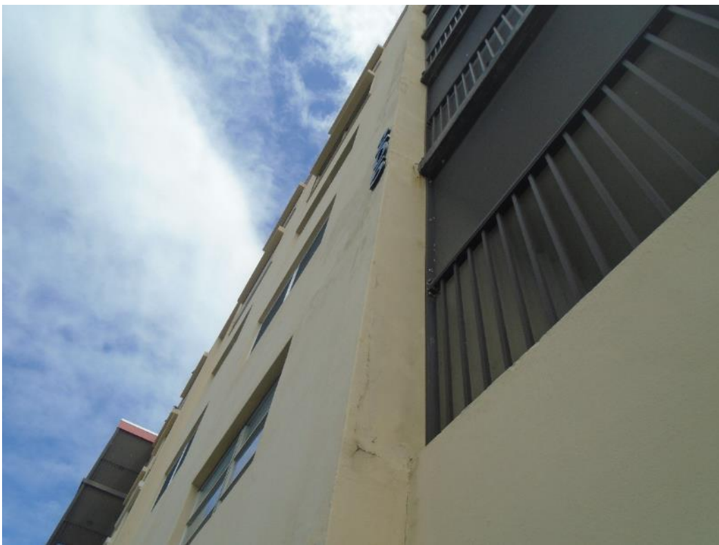
Example view Column Concrete spalling due to reinforcing steel corrosion
