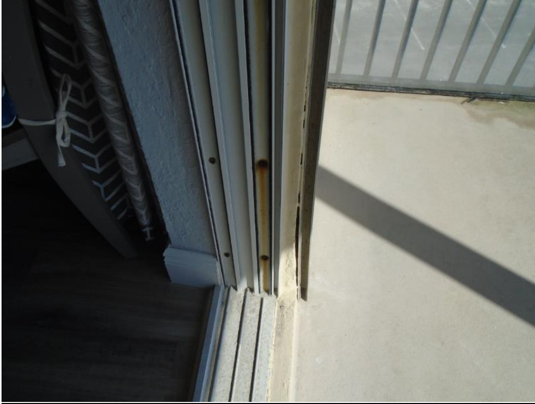
Example view of corroding sliding glass door fasteners
