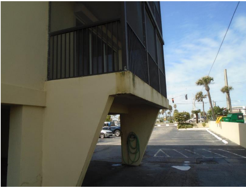
Example view of stucco and paint damage due to inhibition of balcony drainage at screen frame tracks
