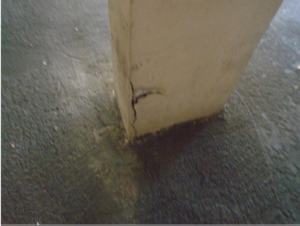
Example view Garage Column Concrete spalling due to reinforcing steel corrosion
