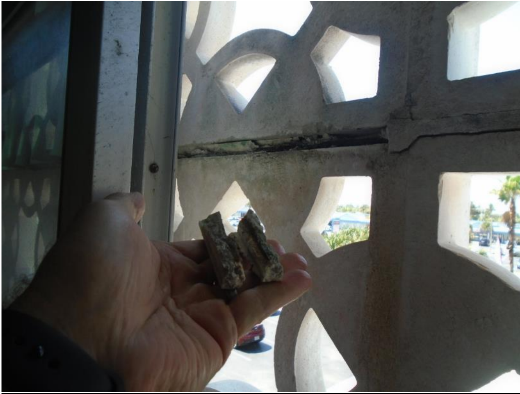
Example view of decorative block deterioration and corrosion
