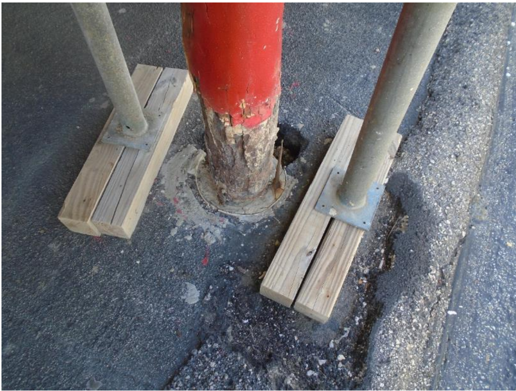
Example view of corroded steel garage support columns
