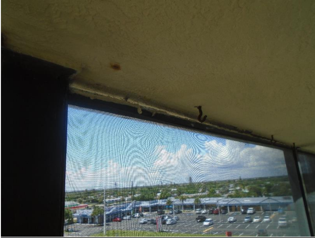
Example view of screen frame fastener deterioration
