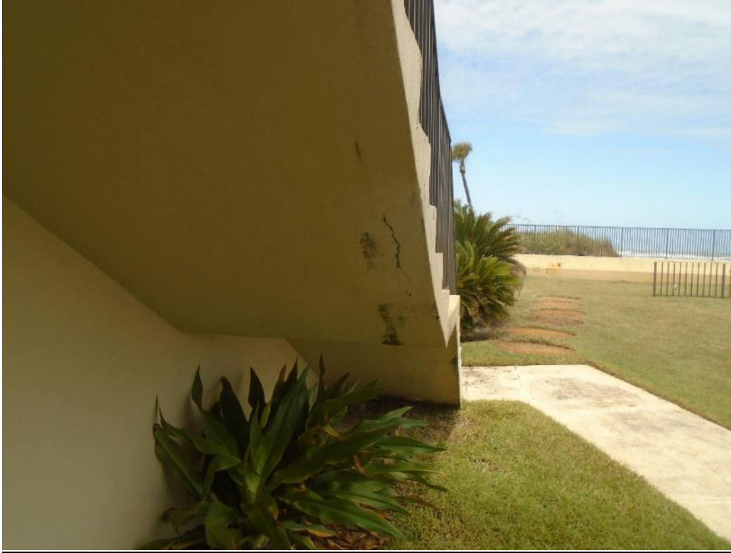
Example view Stairs Concrete spalling due to reinforcing steel corrosion
