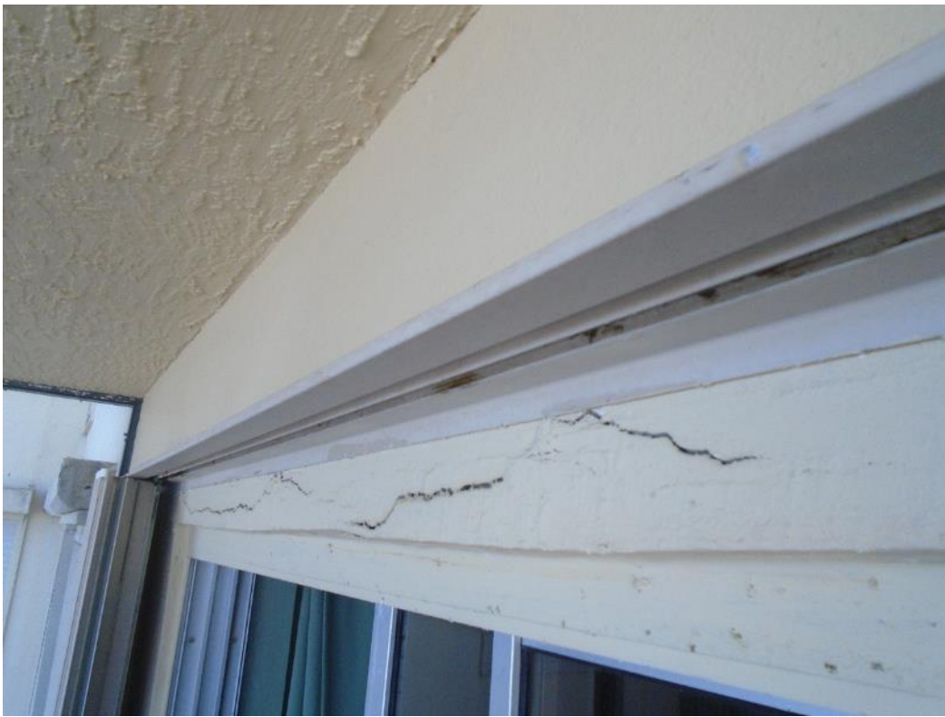
Example view Sliding Glass Door Header Beam Concrete spalling due to reinforcing steel corrosion
