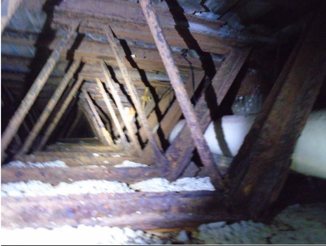
Example view of corroded substructure under northeast garage roof balconies
