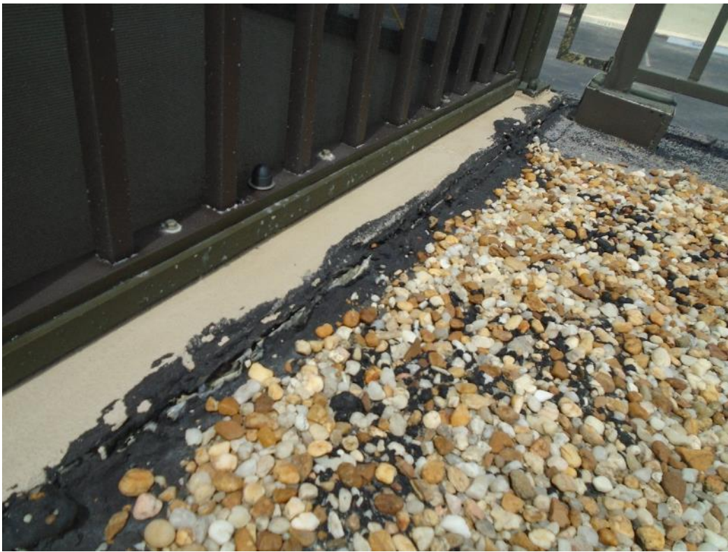
Example view of questionable flashing at roof mounted balcony over garage
