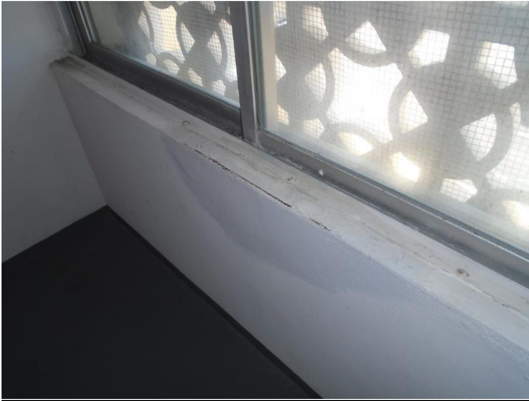
Example view of water intrusion damage behind decorative block windows
