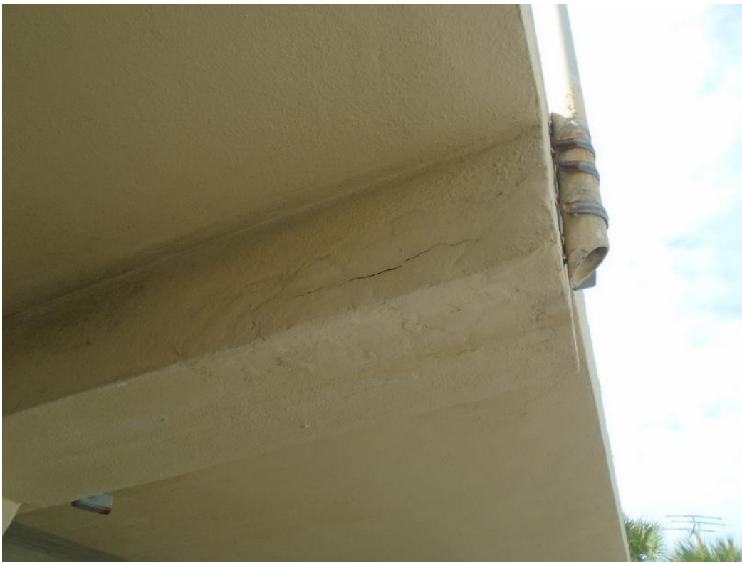
Example view Beam Concrete spalling due to reinforcing steel corrosion-with past repairs in failure
