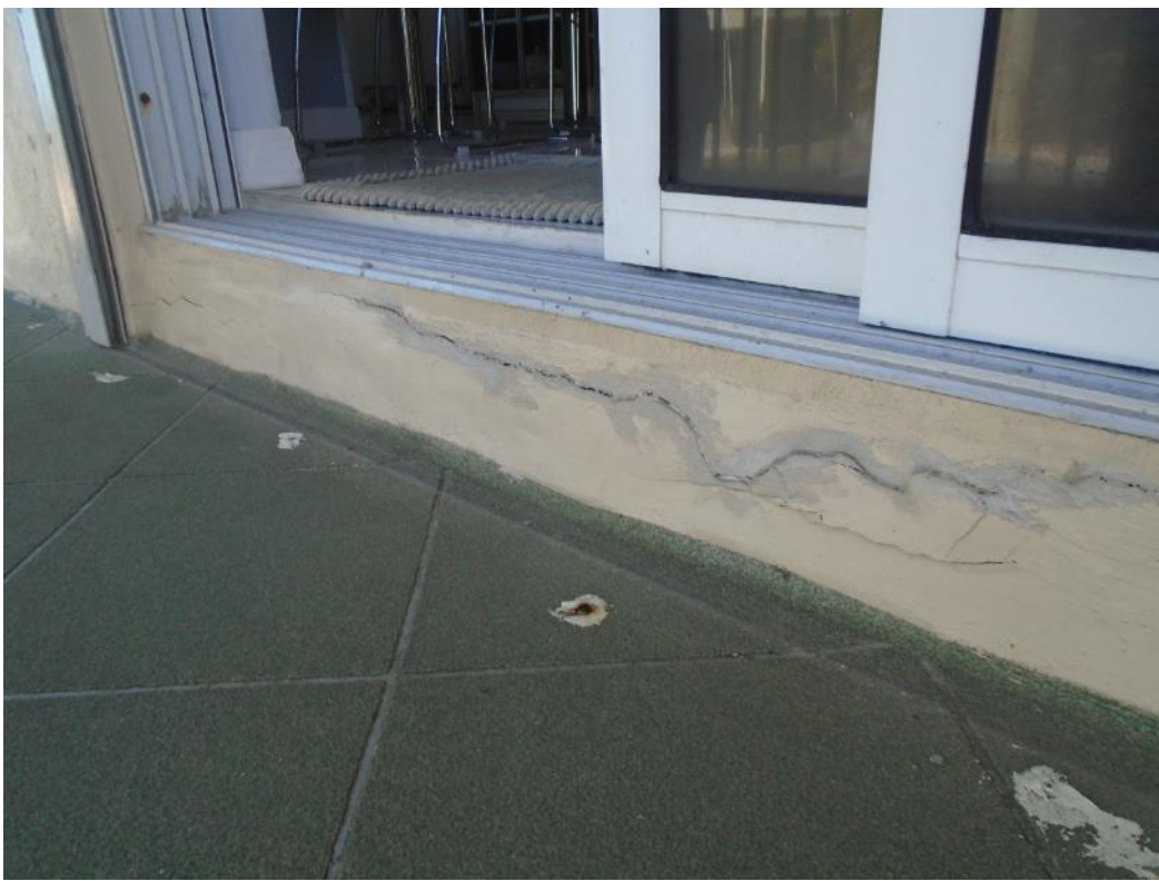
Example view Sliding Glass Door Sill Concrete spalling due to reinforcing steel corrosion
