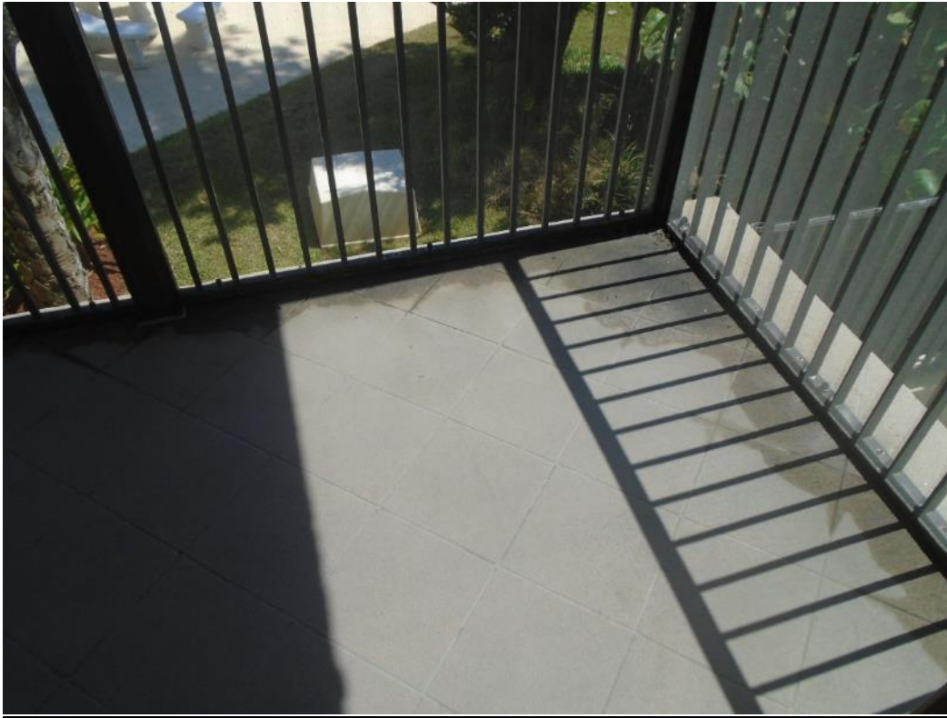
Example view of balcony drainage inhibited by the screen framing
