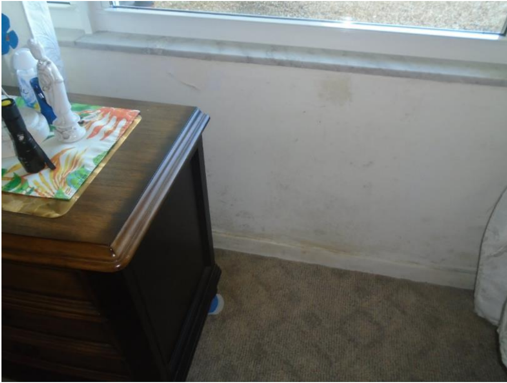
Example view of water intrusion at window opening due to either window failure, sealant failure or structural damage
