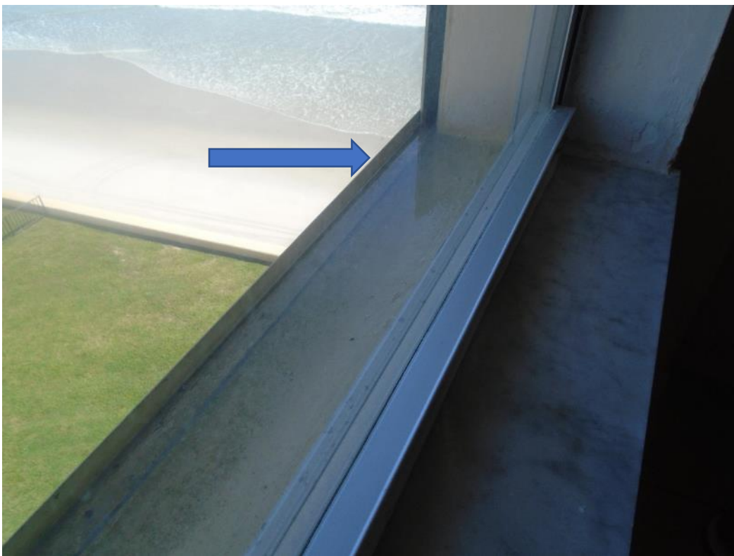
Example view of window shutter track inhibiting drainage off of sill
