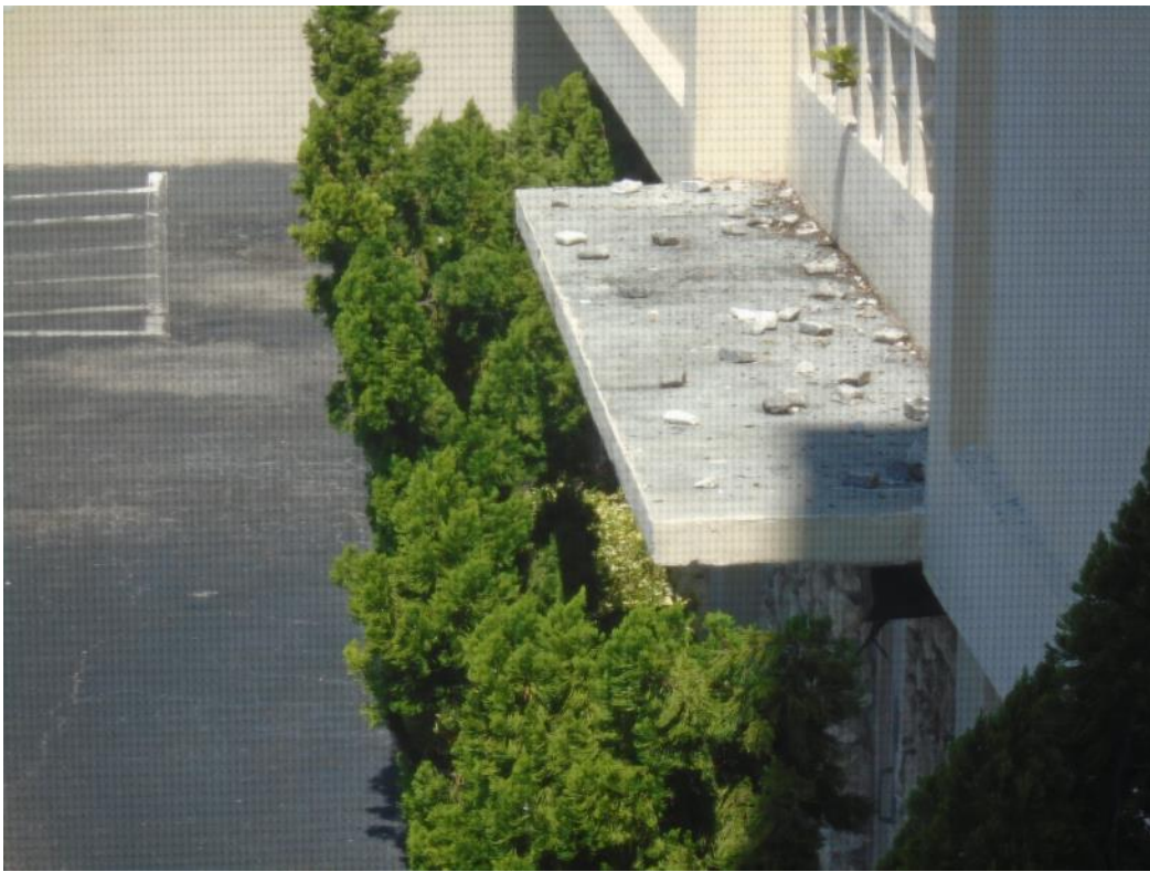
Example view of falling debris from decorative block deterioration
