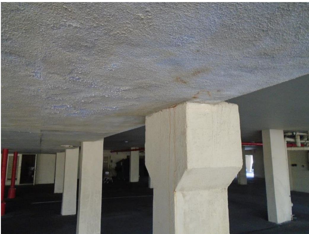
Visual evidence of long term water intrusion from northeast garage roof under balconies
