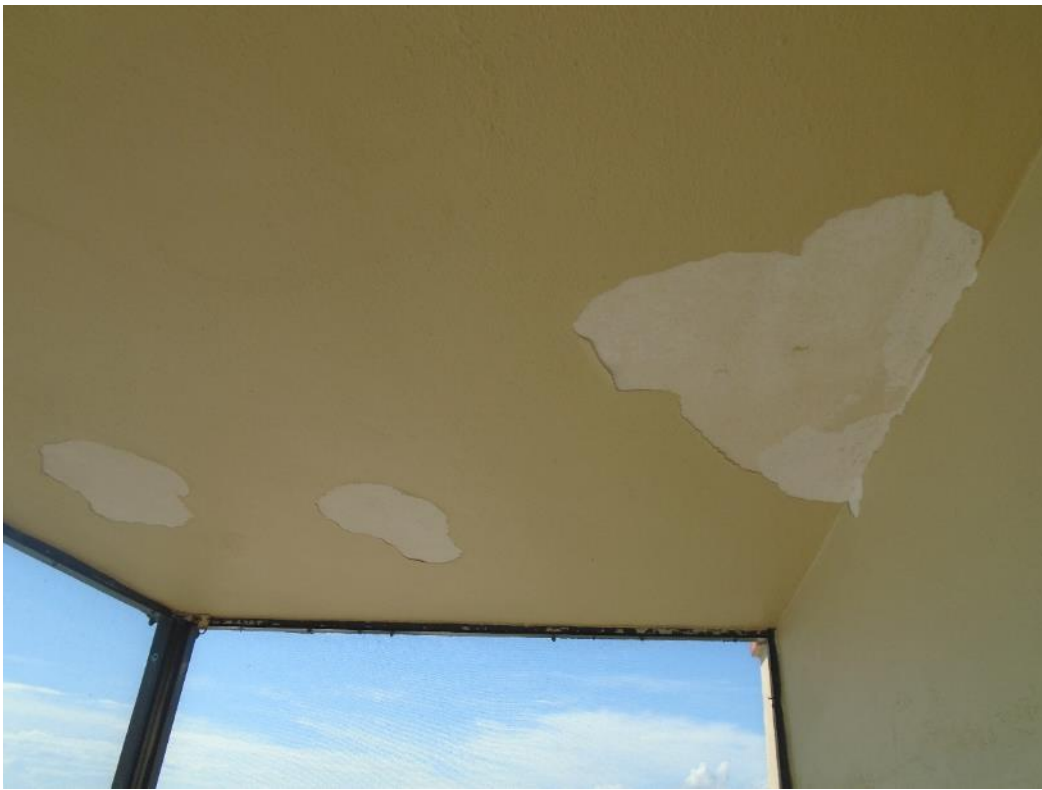
Example view of paint loss of adhesion-improper application of elastomeric on balcony ceilings
