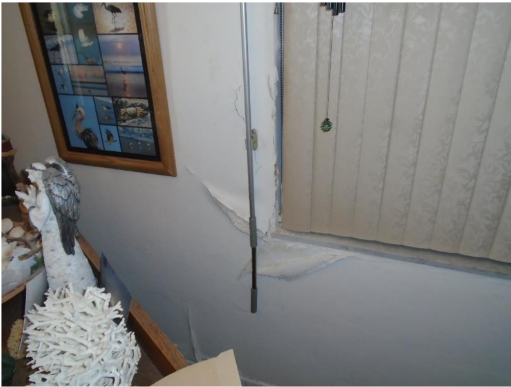
Example view of water intrusion at window opening due to either window failure, sealant failure or structural damage
