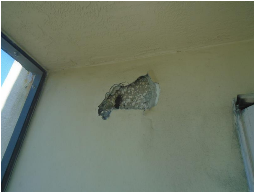
Example view Exposed Wall Concrete spalling due to reinforcing steel corrosion
