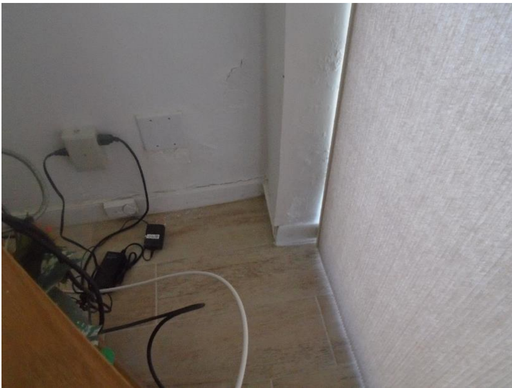
Example view of water intrusion at Sliding Glass Door opening
