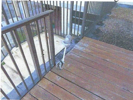
View of damaged light fixture at rear deck stairway
