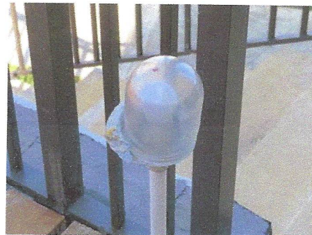
Closer view of damaged light fixture
