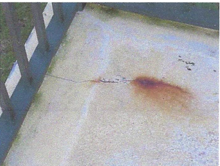
Closer view of spalling condition at landing
