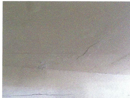
Closer view of spalling conditions
