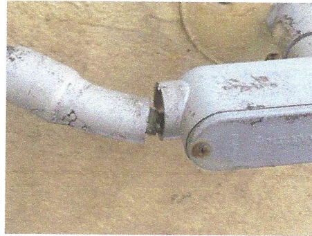
Closer view of disconnected conduit and exposed wiring
