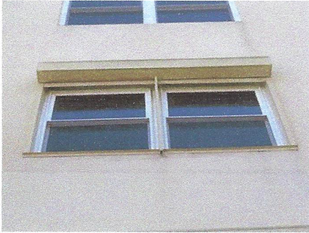
View of exterior north side window with spalling condition at sill below
