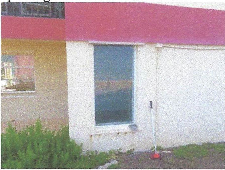
View of exterior east side window adjacent to card room with spalling condition at sill
