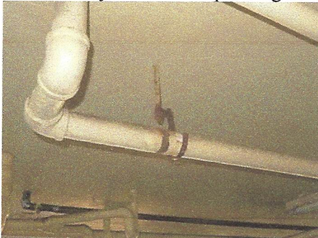
Another view of piping supports which have rusted away in covered parking areas
