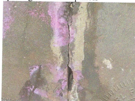
Closer view of typical open joint at seawall face
