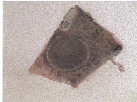
View of typical missing exhaust fan assembly in laundry room restrooms
