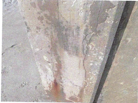
Closer view of typical spalling condition on seawall column
