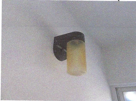
View of damaged light fixture in north stairway at fourth-floor landing
