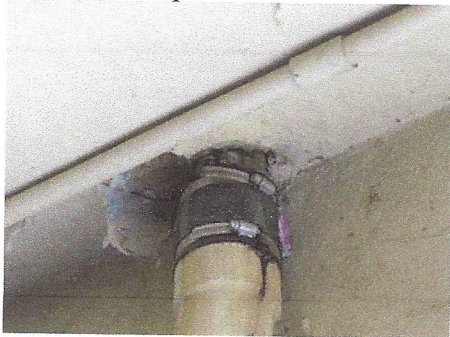
View of typical improper repair evidence and leakage waste piping
