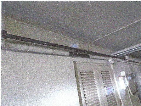
View of typical hydronic supply/return lines in covered parking areas
