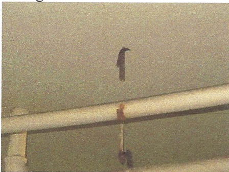
Closer view of piping supports which have rusted away in covered parking areas
