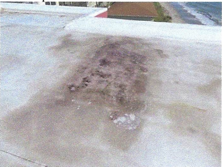
View of typical ponding water and algae development on main roof surfaces
