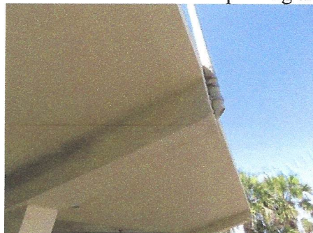
View of spalling evidence at north beam over front carport
