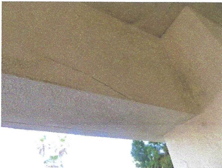
Another view of spalling conditions at beam
