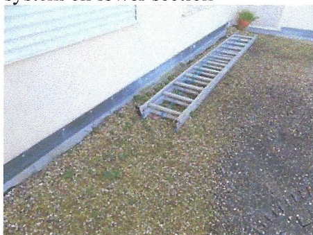
View of typical ponding water and algae development on lower roof surfaces
