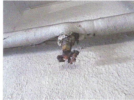
Another view of typical nonfunctional shut-off valve with deteriorated valve handle at hydronic piping in covered garage areas
