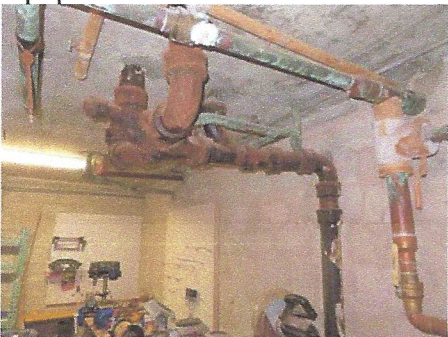
View of typical cast-iron waste piping in boiler room
