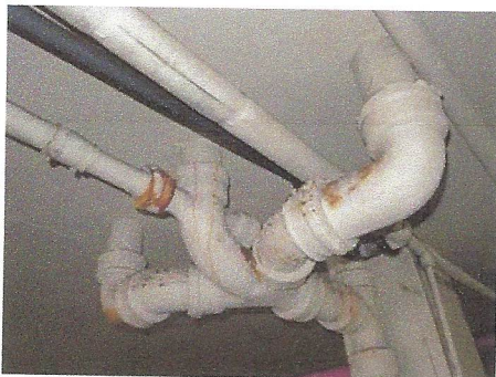
View of typical cast-iron waste piping, from living units, in south covered parking area
