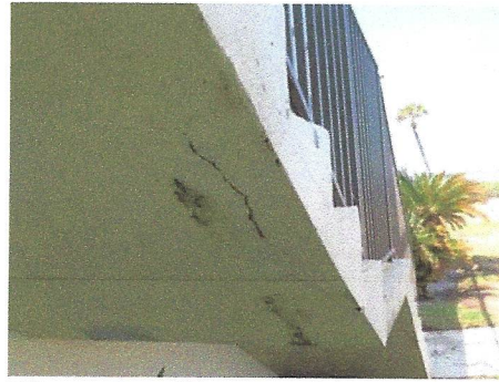
View of spalling condition at underside of stairway
