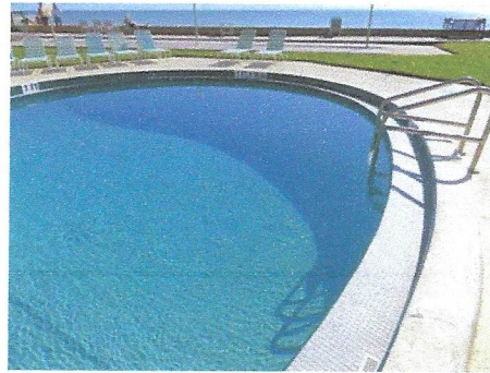
View of perimeter drainage shelf which leaks, as per building maintenance personnel
