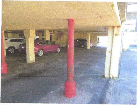
View of typical north covered parking area column with corrosion which needs to be wire brushed and protected with rust inhibitive
