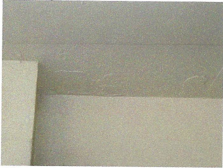
Closer view of spalling condition at ceiling/deck in north covered parking area
