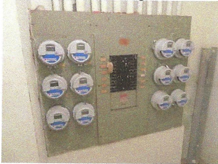
General view of typical meter bank and main disconnects in electrical rooms on most floors
