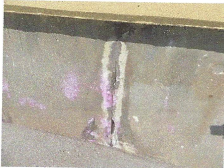
View of typical open joint in seawall panels which need to be properly sealed to prevent washout of backfill
