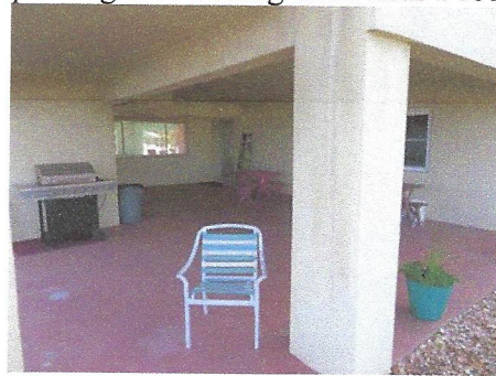
View of barbecue area and column with spalling condition
