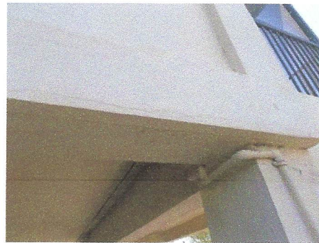
Closer view of spalling conditions
