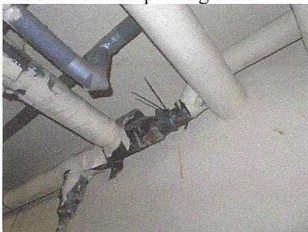
Another view of typical hydronic supply/return lines in covered parking areas
