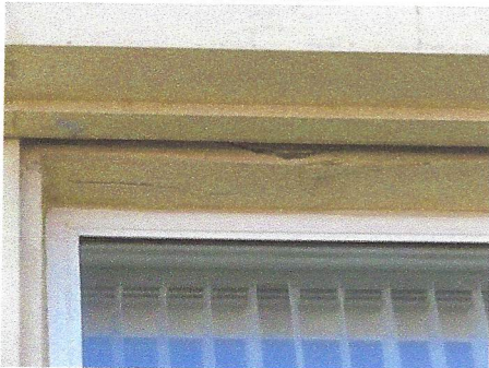
Closer view of spalling condition on header/lintel
