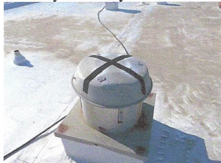
View of typical improper duct tape repairs at ventilation dome/covers
