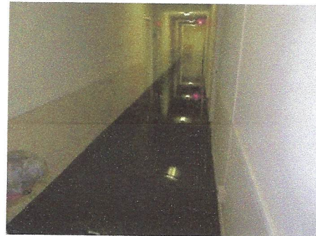
Another view of inundation on fourth-floor
