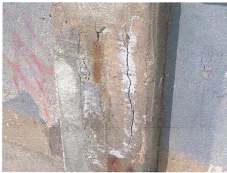
View of typical spalling condition on seawall column
