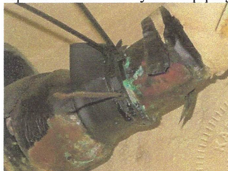
View of typical improper/temporary repairs observed on hydronic piping
