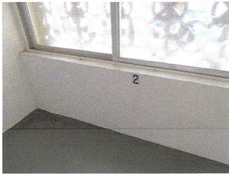
View of typical moisture penetration evidence around window openings in stairway
