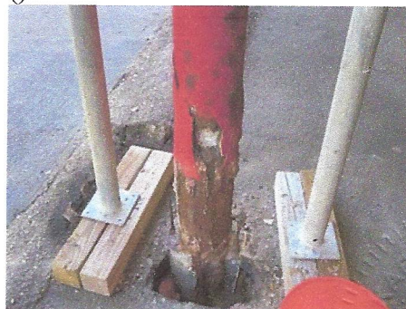
Closer view of column which and foundation which need to be replaced
