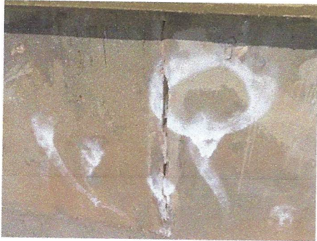
Closer view of typical open joint at seawall face
