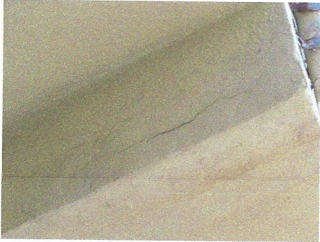
Closer view of spalling evidence and patching
