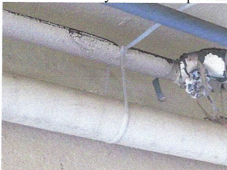
Closer view of improper piping support
