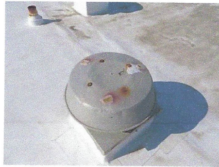
View of typical ventilation dome/cover which has rusted through and allows moisture intrusion into the structure
