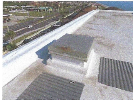
View of north roof access hatch with latch that has broken off
