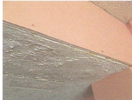
Closer view of leakage evidence which occurs due to back-ups in cast-iron waste piping
