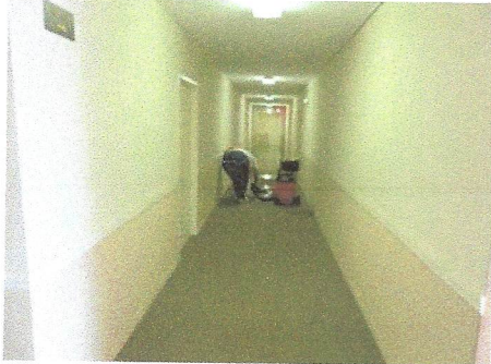
View of inundation which occurred in fourth-floor south corridor due to leakage from air handler unit hydronic lines
