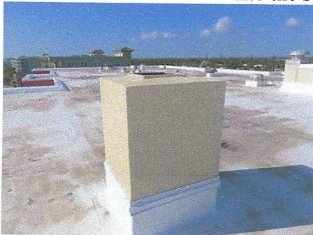
View of chimney at mid-east rooftop area which does not have a rain cap
