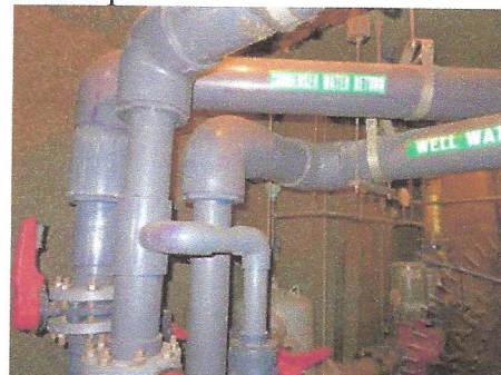
View of hydronic piping in mechanical room
