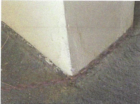
View of spalling conditions at base of column in south covered parking area
