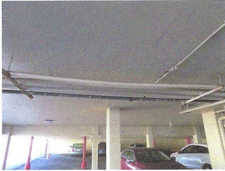
View of unsupported waste piping in north covered parking area
