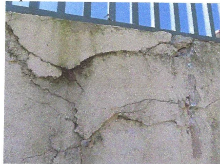
Closer view of spalling evidence at north side cap
