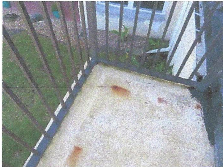
View of spalling condition at upper stairway landing
