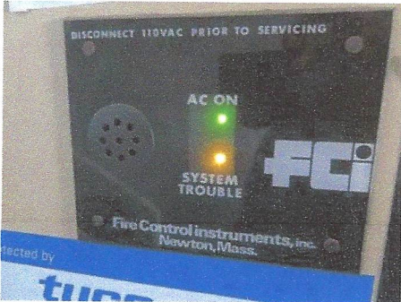
View of "System Trouble" code displayed on fire alarm control panel
