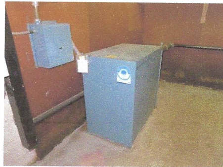
View of east elevator hydraulic system
