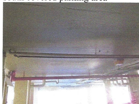
View of unsupported waste piping in north covered parking area
