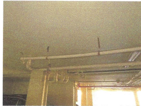
View of typical piping supports which have rusted away in covered parking areas
