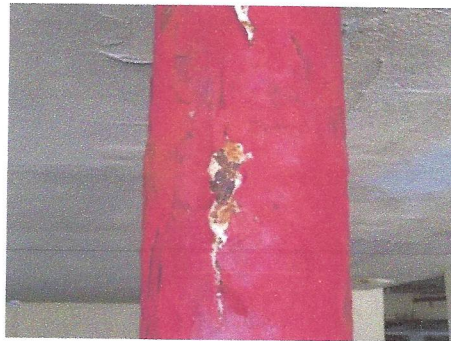
Closer view of typical corrosion on north covered parking area columns
