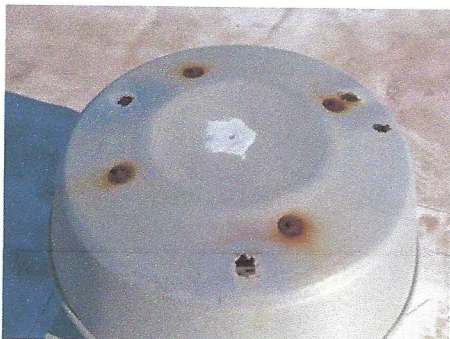
Another view of typical ventilation dome/cover which has rusted through and allows moisture intrusion into the structure
