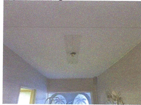
View of open junction box and exposed wiring at ceiling in lobby area
