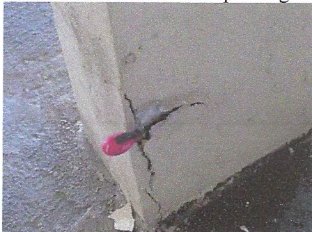
Closer view of spalling condition at base of column in south covered parking area
