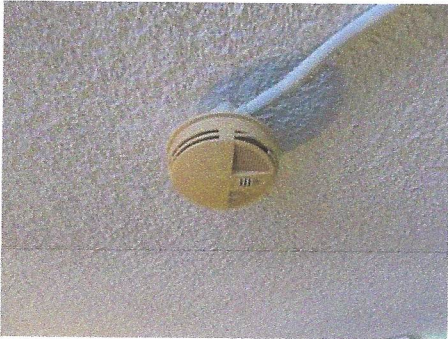
View of typical smoke detector device in hallway corridors which has exceeded its useful service life
