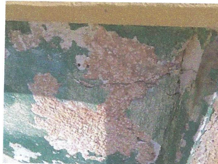
View of typical cracks associated with spalling at seawall panels
