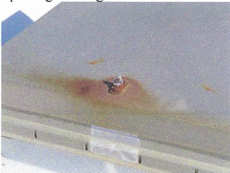
Closer view of latch that has broken off
