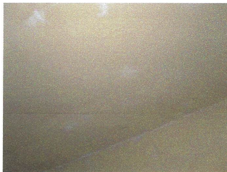
Closer view of spalling conditions
