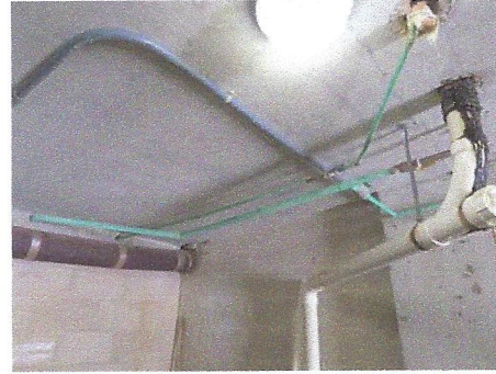
View of unsupported supply piping in pool equipment room
