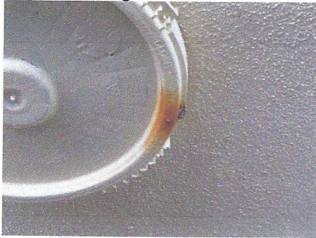
Closer view of leakage evidence through improvised light fixture cover
