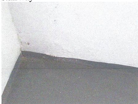
Closer view of moisture penetration evidence
