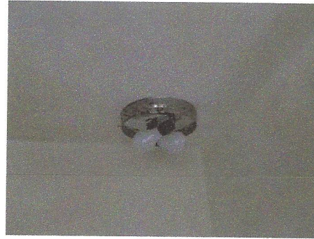
View of typical missing cover at laundry room restroom light fixtures
