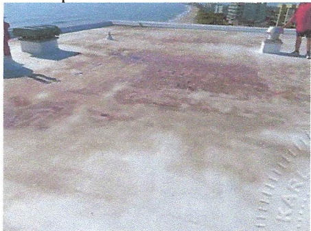
View of typical ponding water and algae development on main roof surfaces
