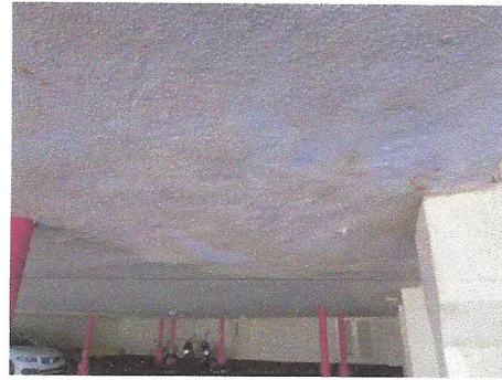
View of typical leakage evidence (water stains) observed at ceiling areas over covered parking
