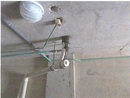
View of leakage evidence at PVC waste line connection to cast iron in pool equipment room
