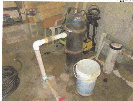
View of abandoned cartridge filter
