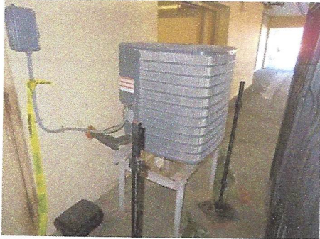
View of condensing unit for elevator equipment room
