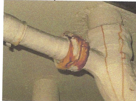
Closer view of leakage evidence from cast-iron waste piping
