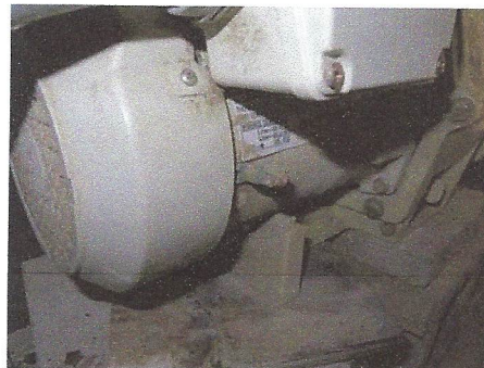
View of missing external bonding wire at pool pump motor
