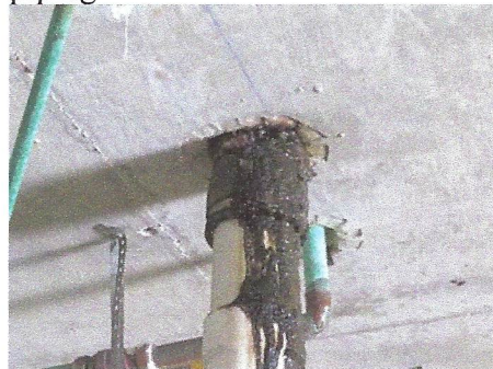
Closer view of leakage evidence
