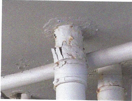
View of typical heavily corroded/deteriorated cast-iron waste piping and repairs evidence
