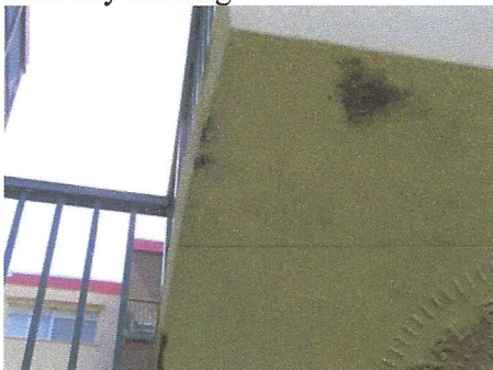
View of spalling condition at edge of landing
