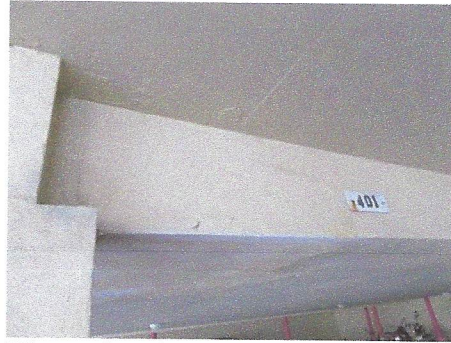
View of spalling condition at north covered parking area ceiling/deck near #401
