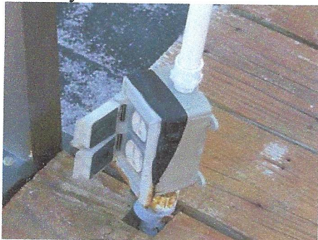
View of receptacle weatherproof cover with improper tape repair and absence of ground fault protection
