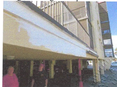
View of reemergence of leakage evidence along north edge after previous refinishing
