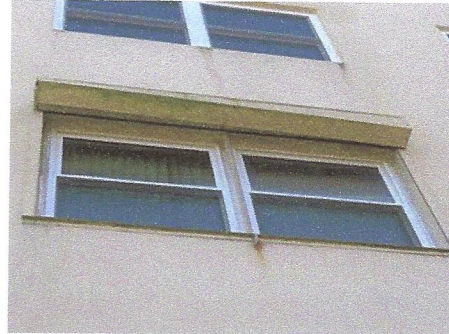
View of typical exterior north side window with spalling condition at header/lintel
