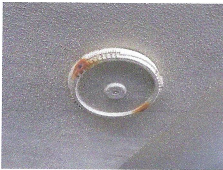
View of leakage evidence through improvised light fixture cover
