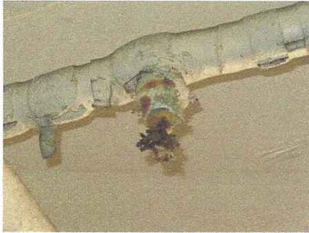
View of typical nonfunctional shut-off valve with deteriorated valve handle at hydronic piping in covered garage areas
