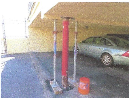
View of north covered parking area northeast column which has rusted through and needs to be replaced
