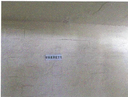
View of spalling condition at ceiling in covered parking area near "Garrett" parking space
