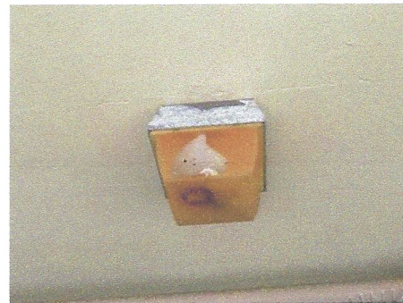
Another view of typical damaged light fixture cover in south covered parking area
