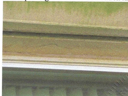
Another view of spalling condition on header/lintel
