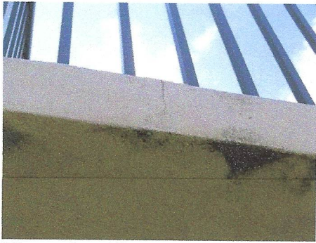
View of spalling condition at edge of landing
