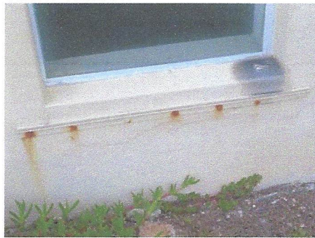
Closer view of spalling condition on sill below window
