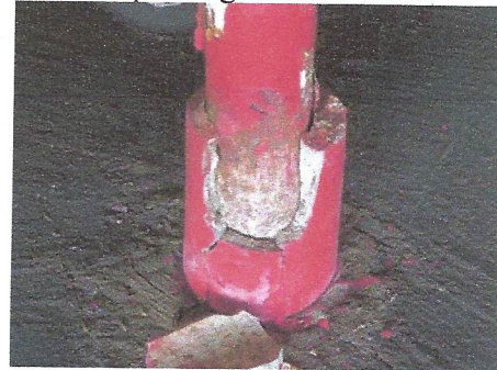
Closer view of typical corrosion on north covered parking area column
