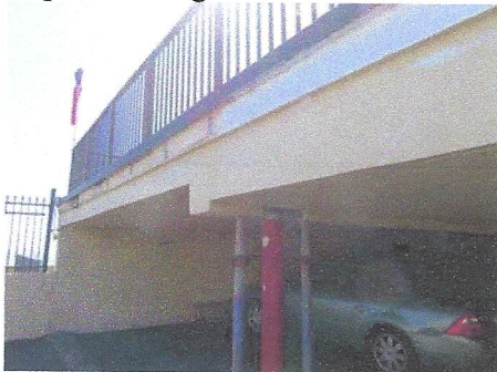
View of reemergence of leakage evidence along north edge after previous refinishing
