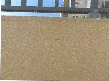
View of spalling evidence at seawall cap at east side
