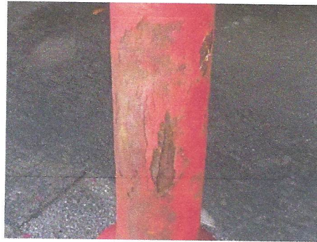
Closer view of typical corrosion on north covered parking area columns
