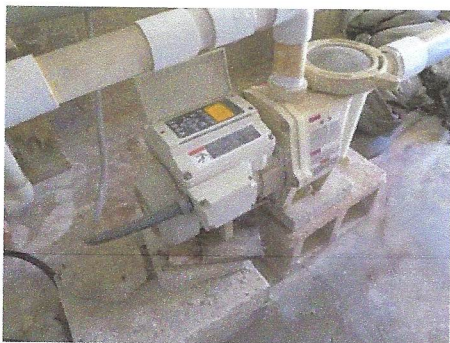
View of pool recirculating pump
