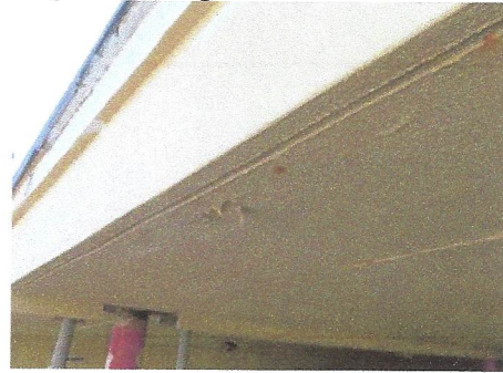
View of reemergence of leakage evidence along north edge after previous refinishing
