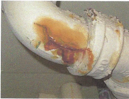
View of typical cracked and deteriorated cast-iron waste piping with evidence of leakage
