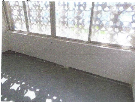
View of typical moisture penetration evidence around window openings in stairway
